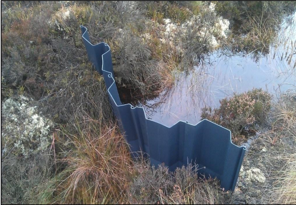
Plate 7. An example of a recycled plastic dam used to block functioning drains on a raised bog site.
